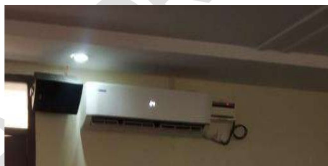
Plate 1: Air conditioning system in Campus
