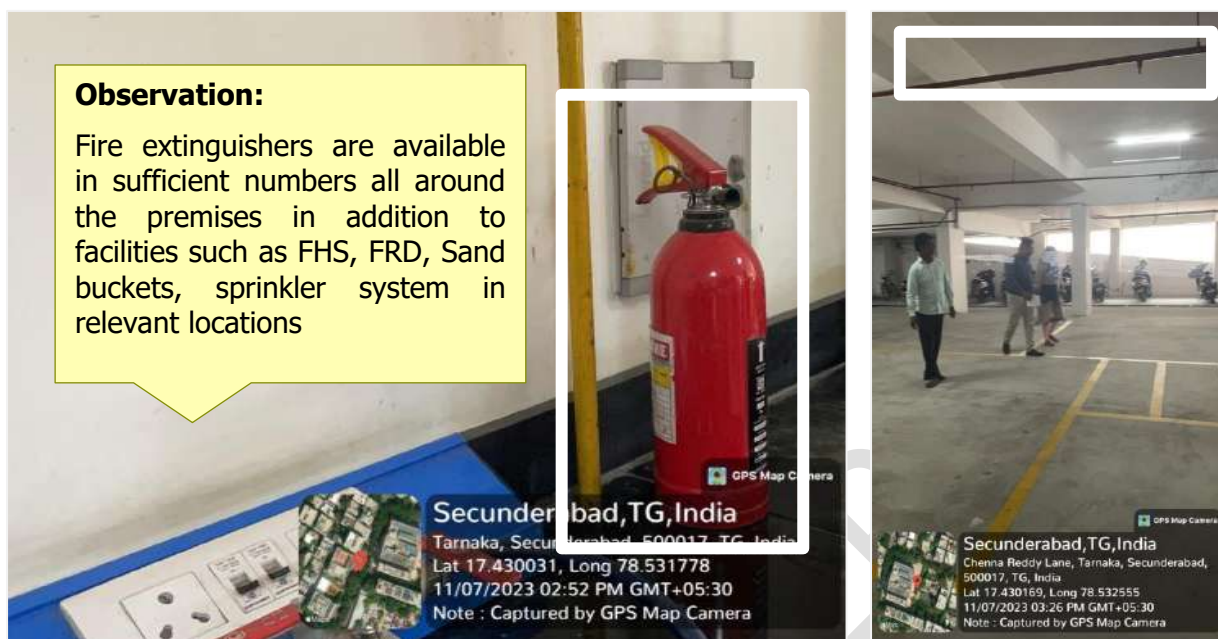
Plate 4: Fire and Life safety practices in the premises
