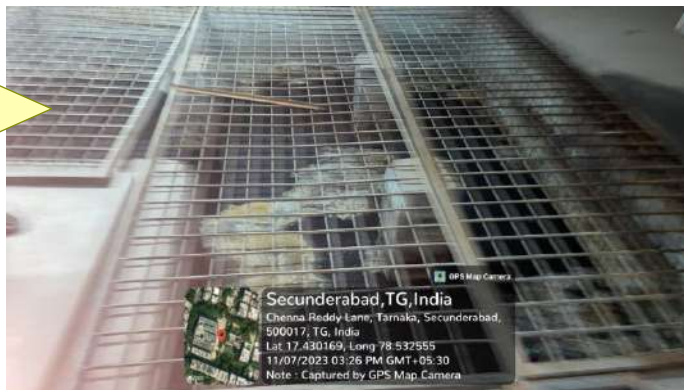
Plate 5: Waste water collection area in the cellar area
